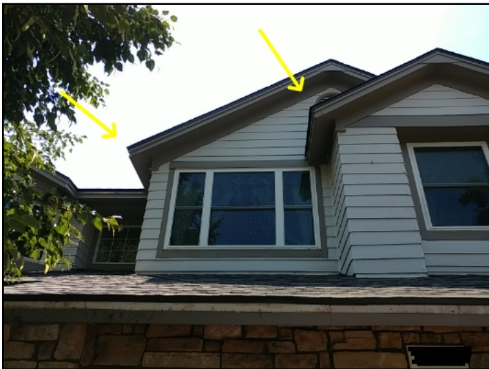
Soffit Corners could use some paint. Front of house.
