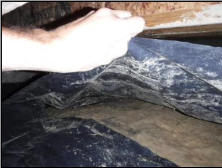
Vapor barrier not sealed at seams or perimeter. Recommend review and repair by qualified contractor.
