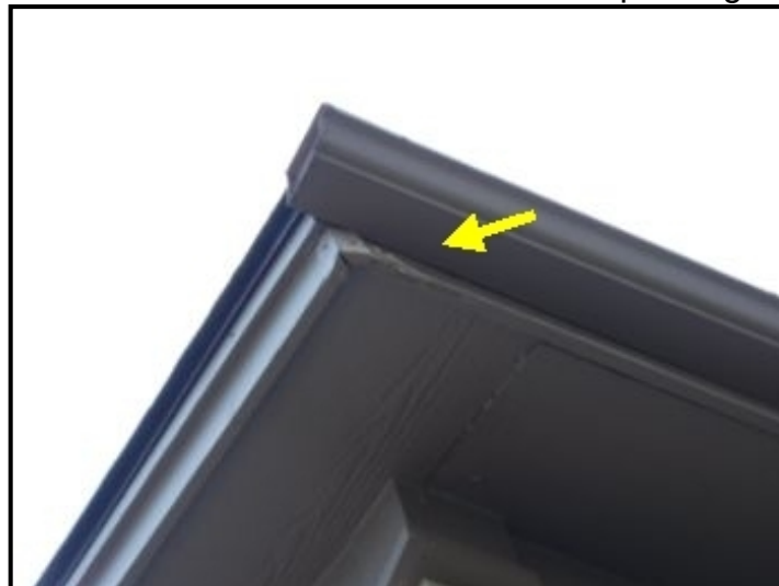
Peeling paint observed, suggest scraping and painting as necessary.
