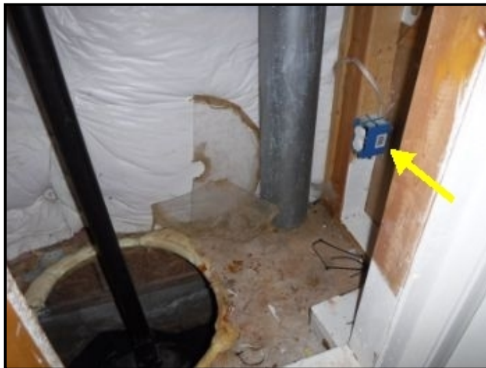
Outlet missing cover plate.
