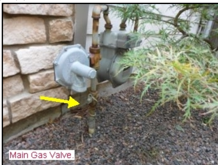
Recommend painting gas pipes to deter rust.
