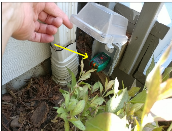
West side of deck by stairs: Outlet has open ground recommend review by qualified electrician.
