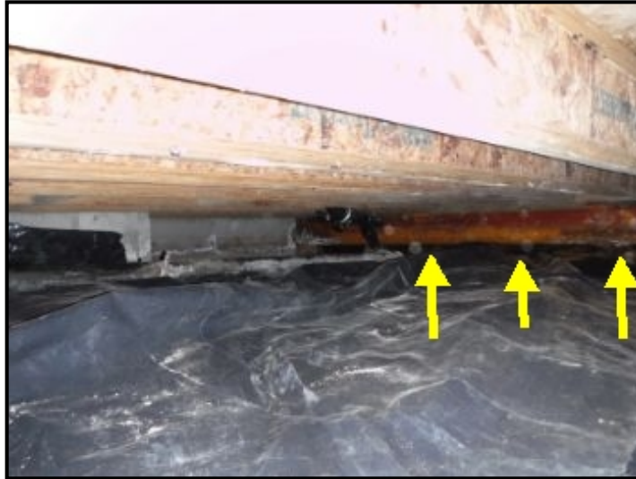
Steel I-Beam is rusted.
