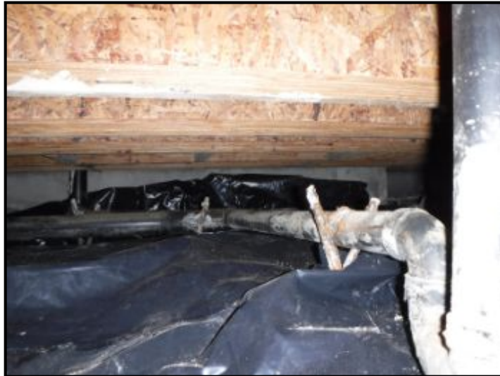
ABS drain pipes need strapping.
