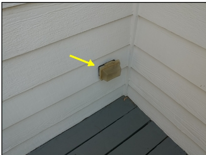
Outlet is loose. West deck.
