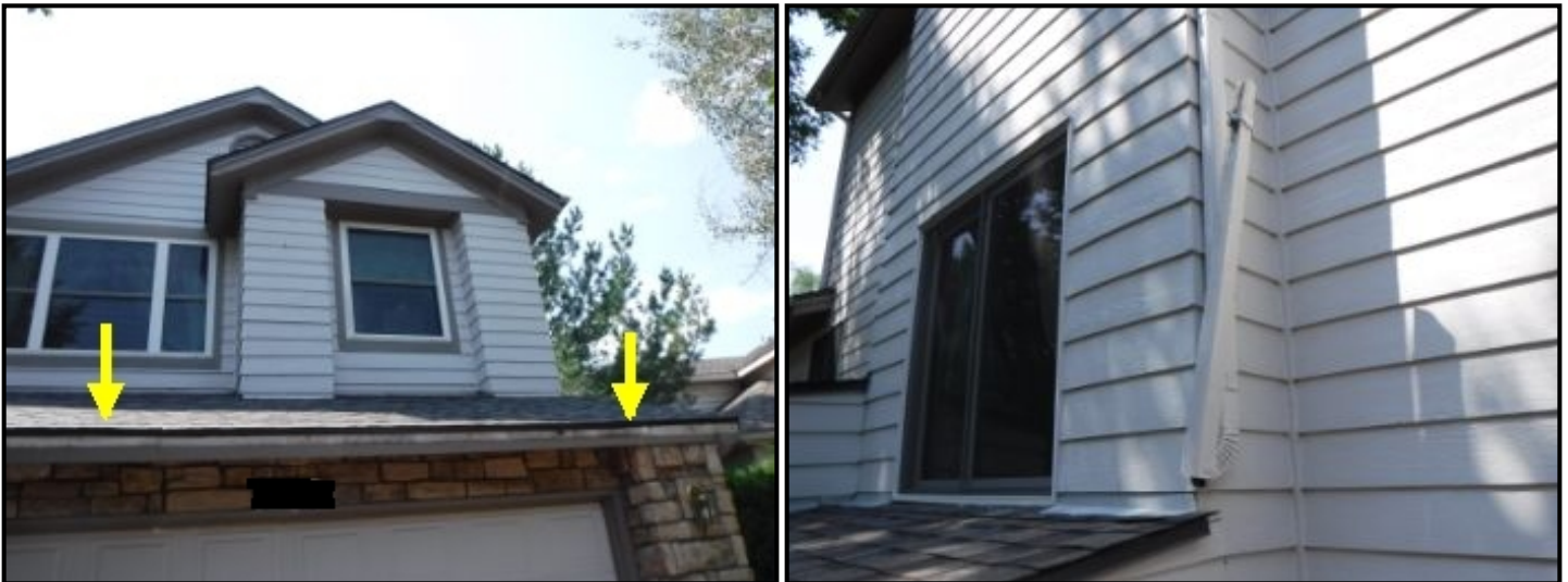
Gutter missing over entranceway to garage; potential ice hazard.
