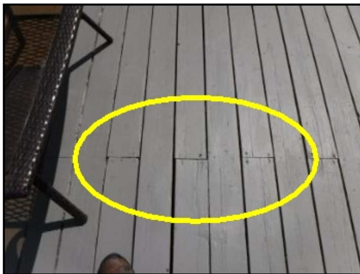
Some deck boards need securing.
