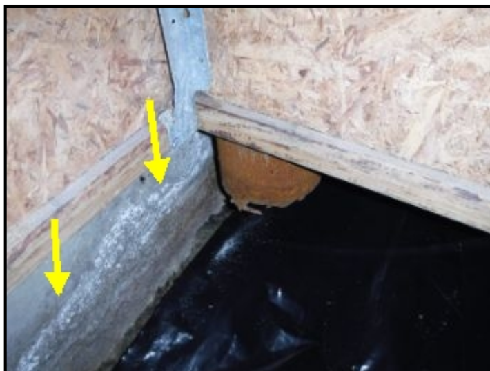
Evidence of past water penetration observed.
