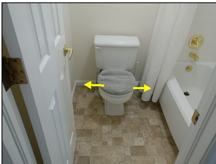
Toilet: East twin bedrooms bath, is loose. Recommend repair by licensed plumber.
